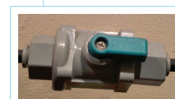
Emergency water shut-off
